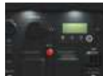
Illuminated Control Panel
